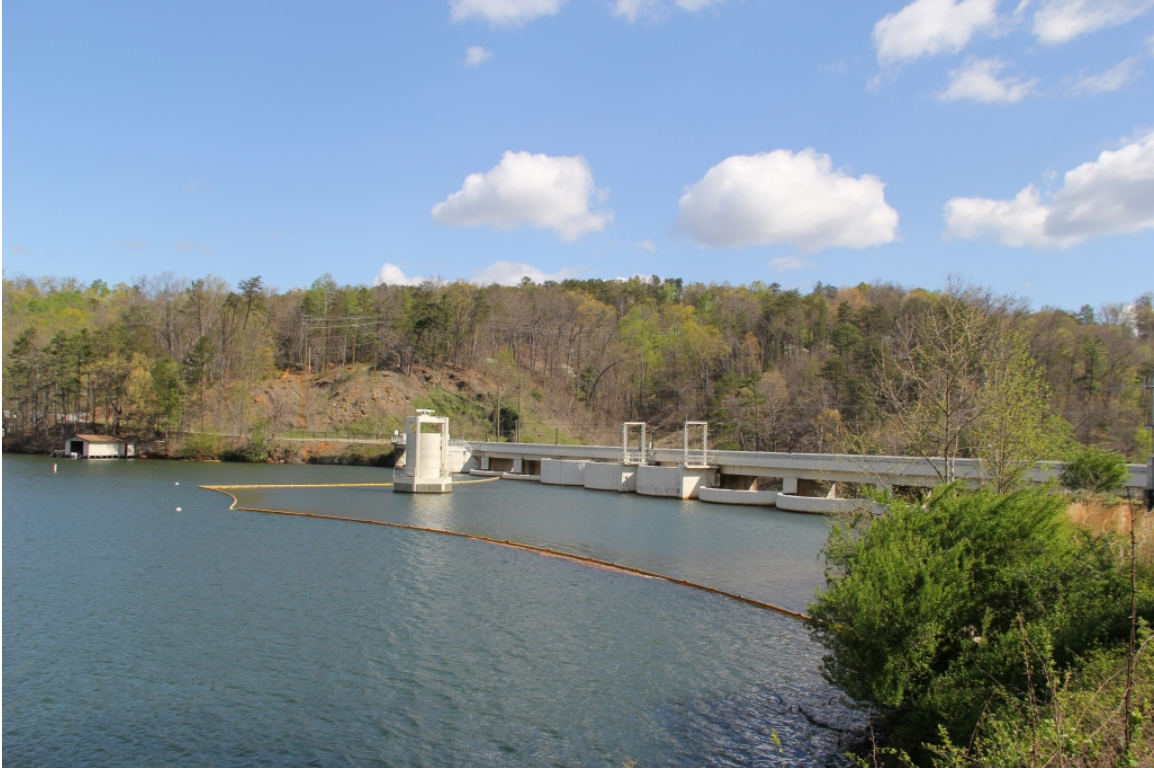
Bridge No. 628 on SR 1306 (Buffalo Shoals Road) over Lake Lure Dam and Broad River, view to northeast
