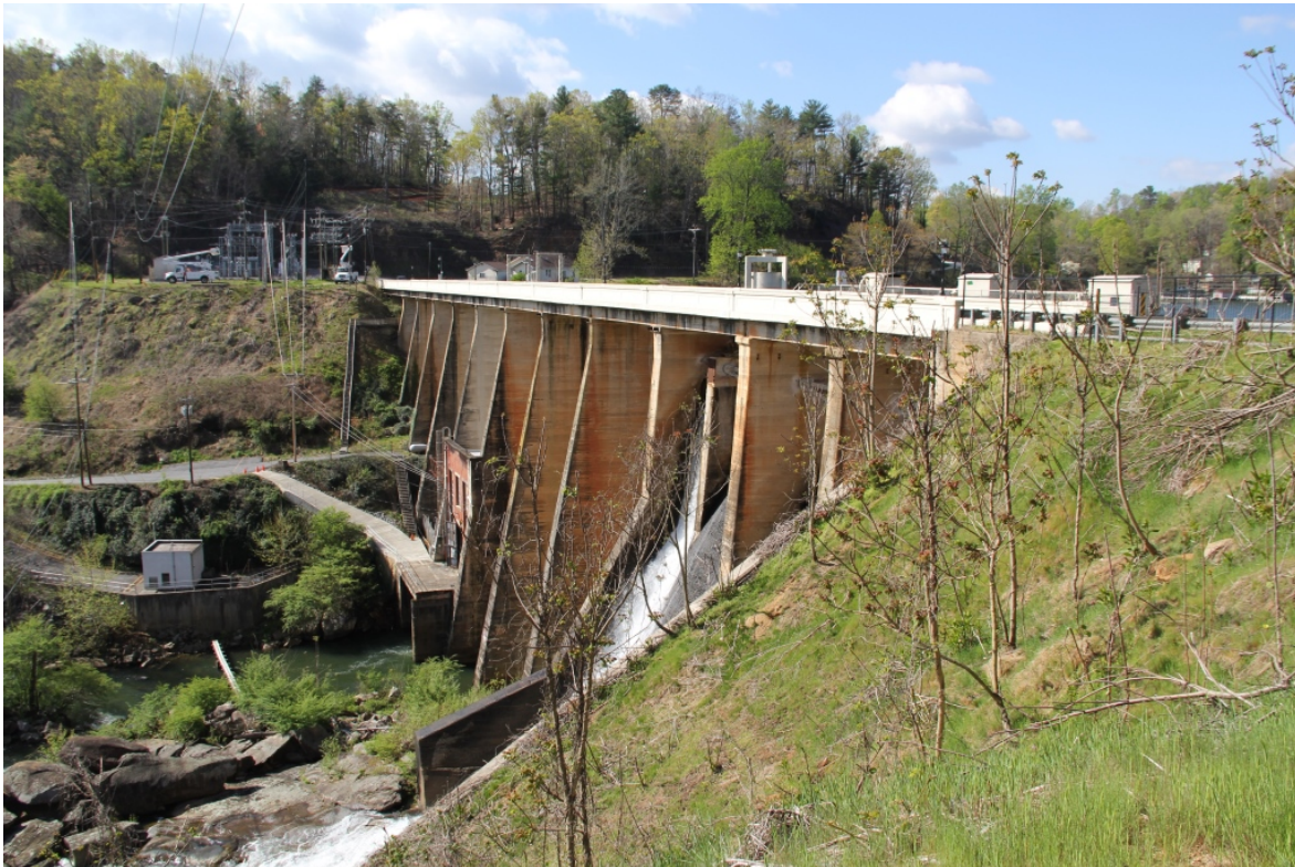
Lake Lure Dam and Hydroelectric Plant, Buffalo Creek Road (SR 1306) over Broad River, oblique view to southwest
