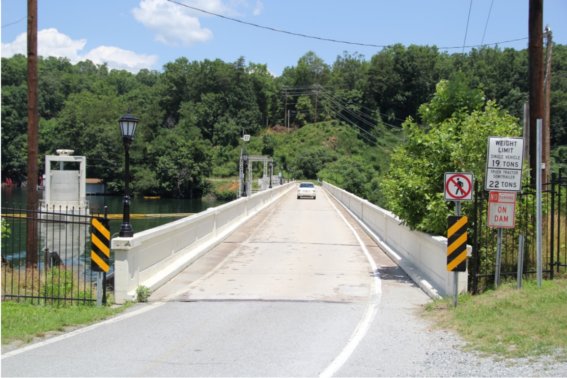
Bridge No. 628 on SR 1306 (Buffalo Shoals Road) over Lake Lure Dam and Broad River, view to north
